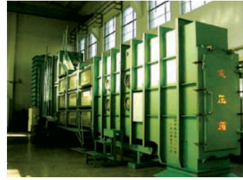
The world's largest vacuum tank (vacuum percentage: 98.7%; flow discharge: 1.0 m 3 /s; maximum working head: 14 m)
