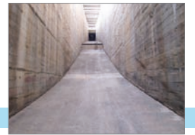
Abrasion resisting concrete with multi-component cementitious powder at the Lijiaxia arch dam
