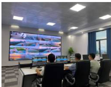
Fig.3 Central Control Room of Shuanggang Navigation Junction
