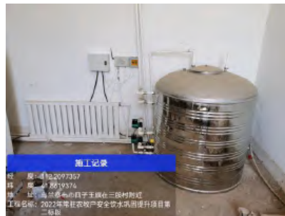
Fig.4 Solar Heating and Anti-freezing Project for Water Purification Room in Ulanqab City, Inner Mongolia
