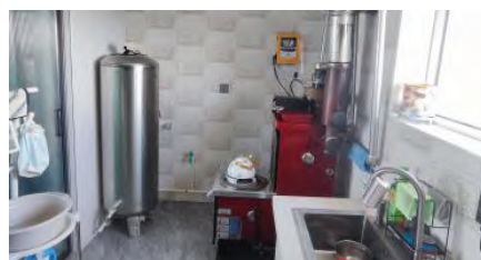
Fig.2 Water Supply to Households Using Photovoltaic Technology and Pressure Tanks in Xilin Gol League, Inner Mongolia
