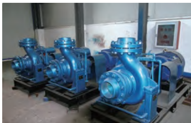
Hot water circulating pump
