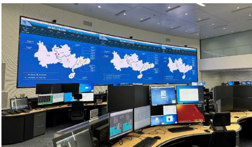
Fig.3 China Southern Power Grid Dual-Regulation Centralized Control Center, China's First Centralized Control System Focused on Pumped Hydro Storage
