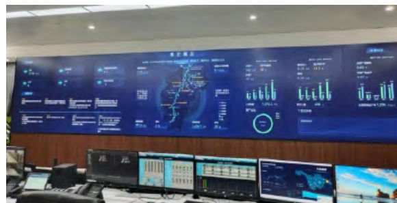
Fig.2 Nanchang Centralized Control Center of JXPG
